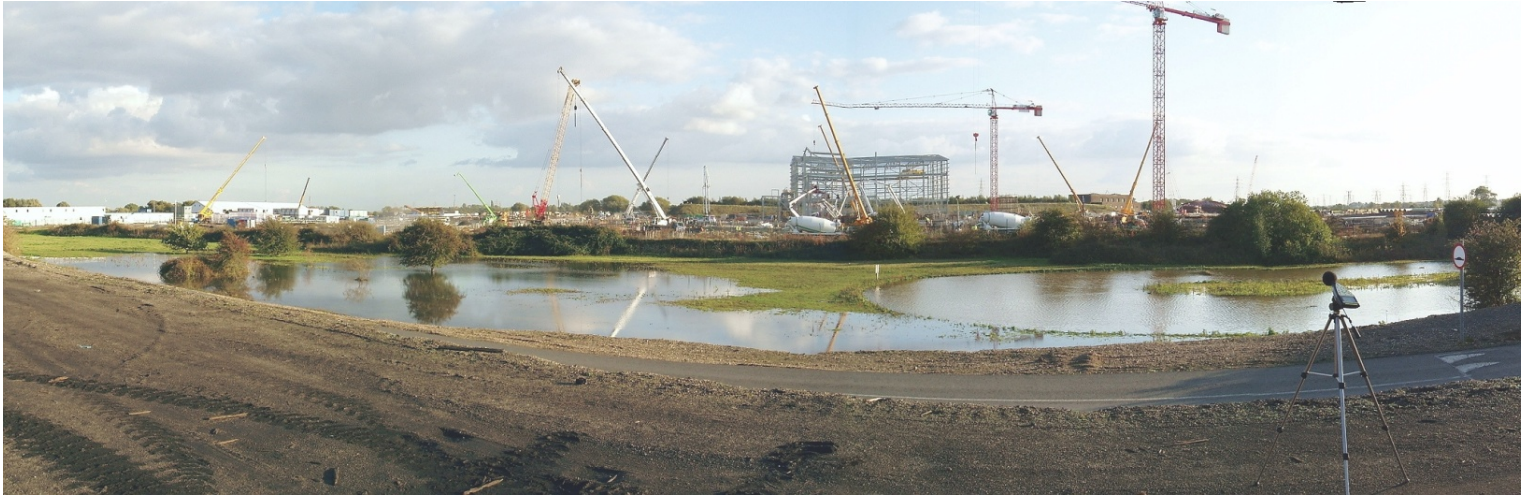
Ongoing noise monitoring during construction of Staythorpe 1650 MWe CCGT Power Station, Nottinghamshire
