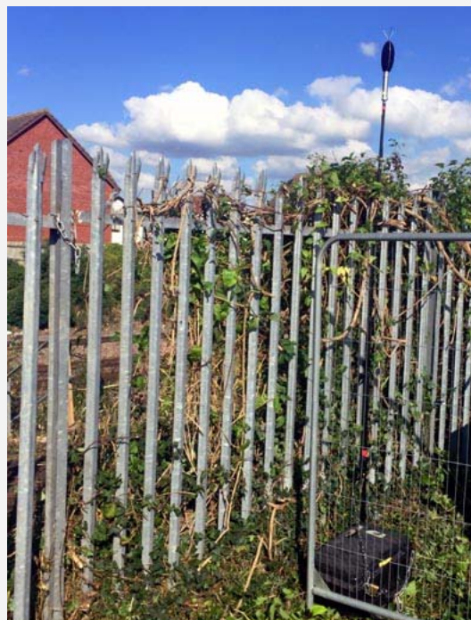
Noise logging equipment at a secure location
